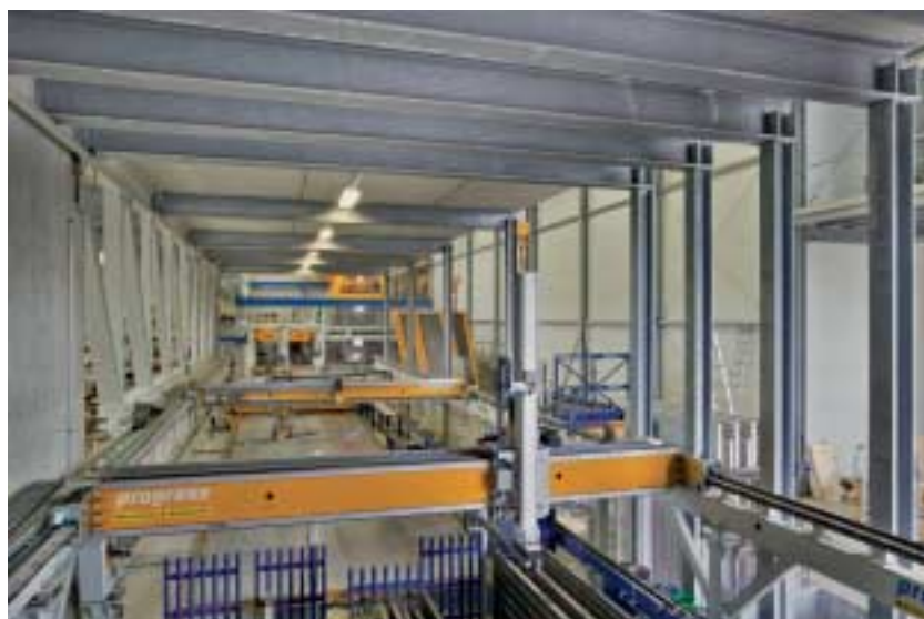
Fig. 4 The shuttering robot does not only serve to move the molds onto the pallet but also to remove them: Molds are lifted from the pallet following a scan procedure. A second robot puts the cleaned molds in store again.
