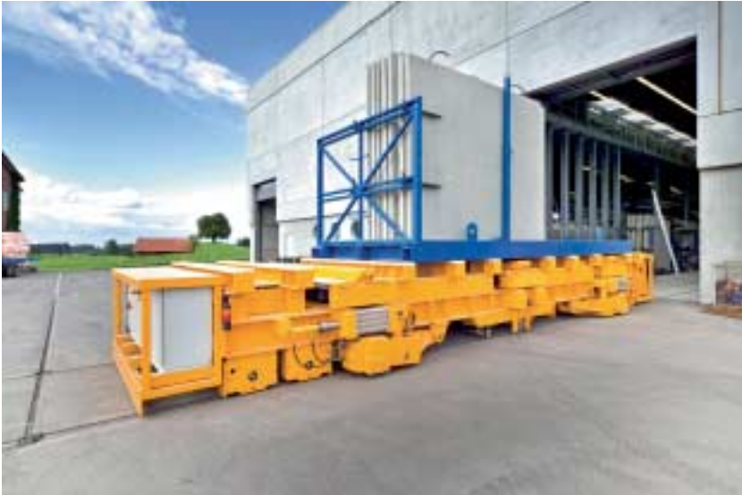
Fig. 11 The produced elements are transported in the outside area with a specially designed exit carriage.
